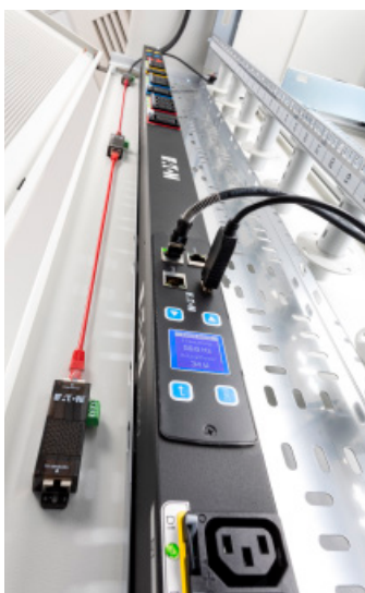
Eaton EMP Gen 2 daisy-chained on rack PDU
